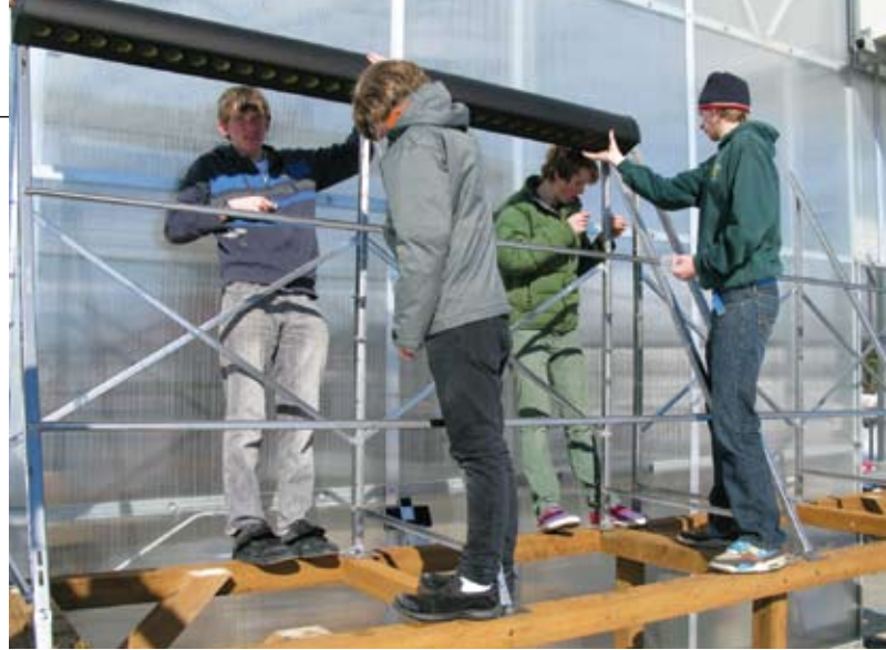
Students install the header for the evacuated tube solar collector as part of the curriculum for the course "Feeding People: The Implications of Agriculture."
